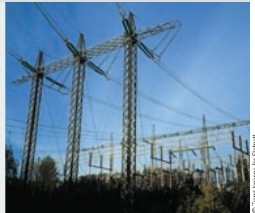
© Trond Isaksen for Statnett
