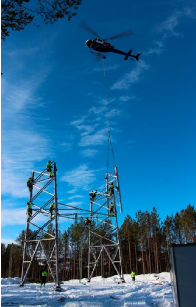
EFFICIENT POWER SUPPLY Construction of a new power line between Balsfjord in Troms County and Skaidi in Finnmark County PHOTO: STATNETT
