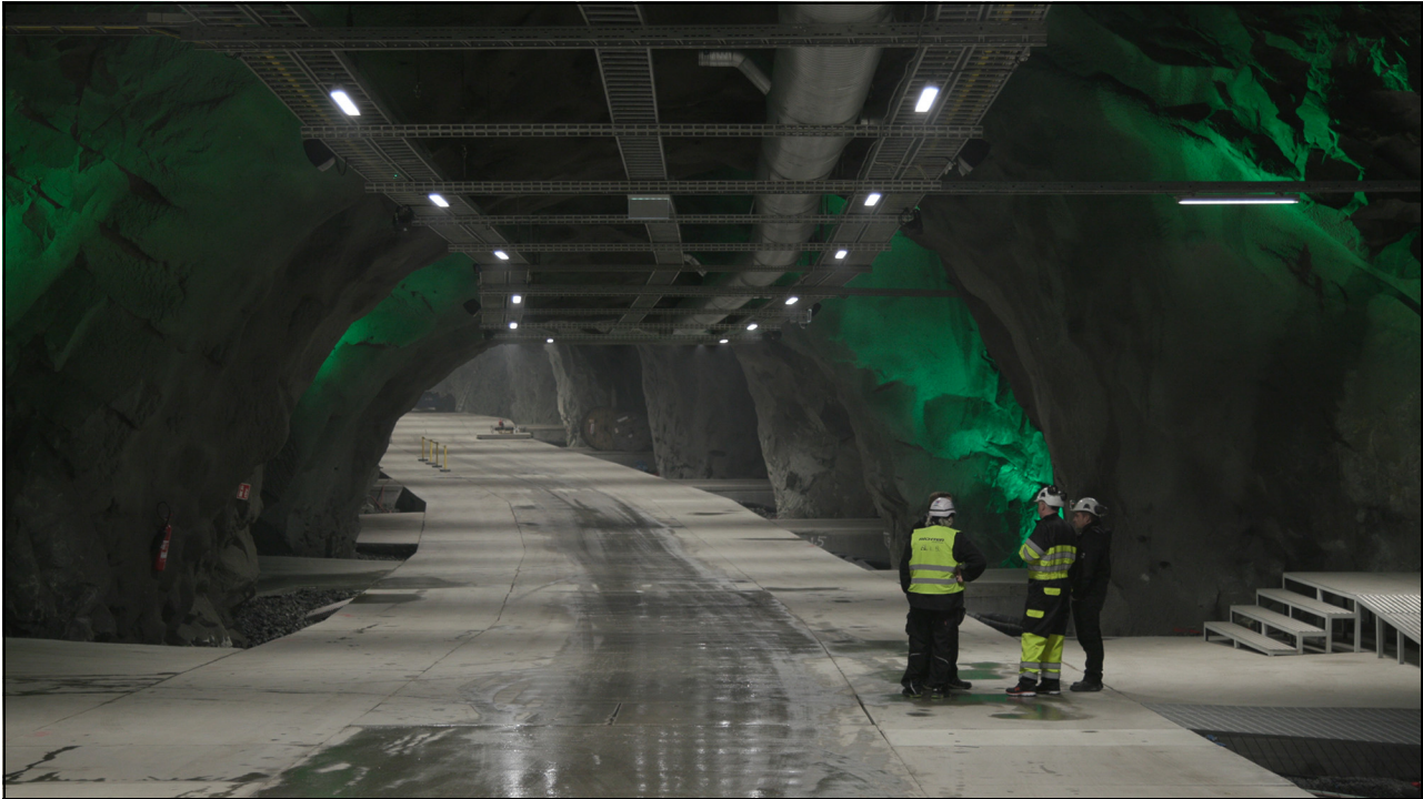
Figure 4.4 Lefdal Mine Data Centre is built in a disused mine between Måløy and Nordfjordeid.
