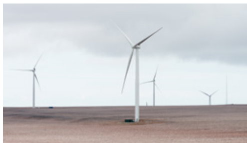
Wind turbines at Raggovidda. Credit: Varanger KraftVind. Photo: Bjarne Riesto
